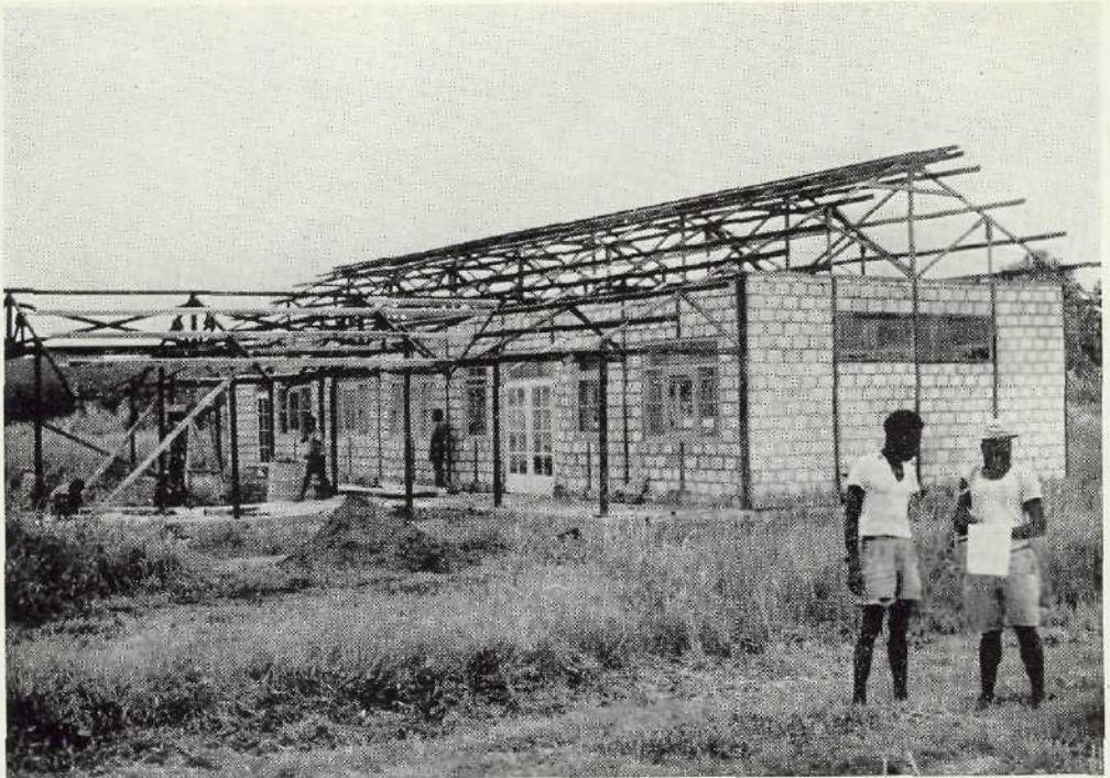
Plate 2. The east-wing of the new hospital under construction. Two Nimboran chief-carpenters are discussing some details.
